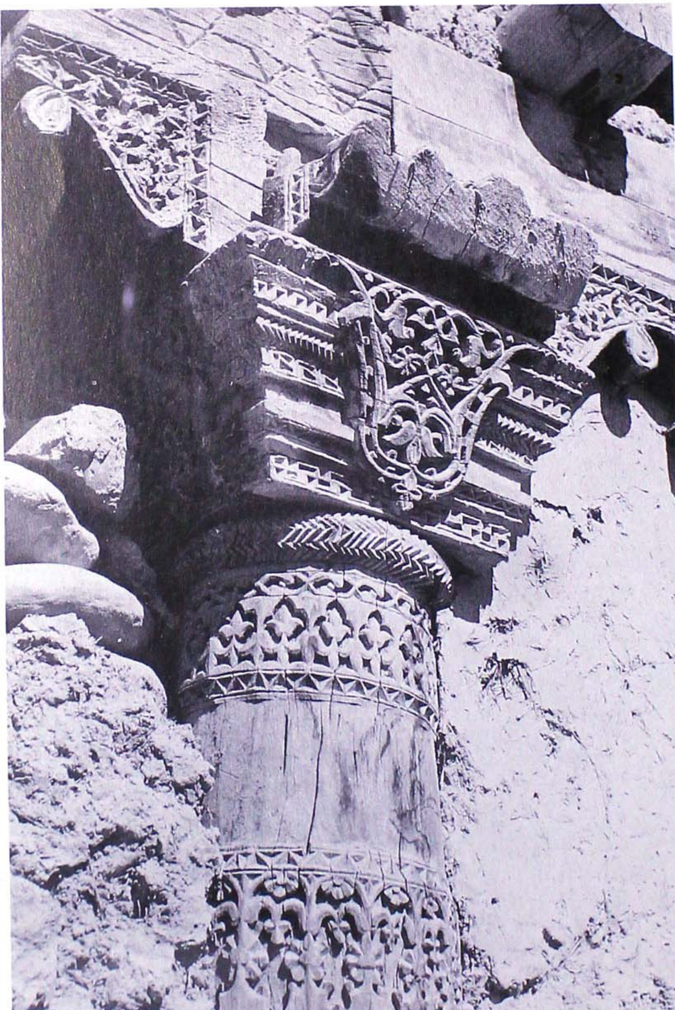
7.38 Timber Column, Skardu. If the rustic brutalism of the structure of this shrine in the remote valley of Shigar appear crude, it is due only to its impoverished state of preservation rather than to a lack of sympathy or respect for the material.
